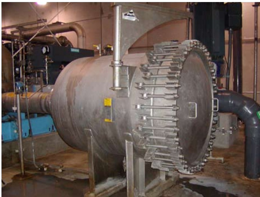
FIGURE 13 Zeron 100 filter vessel for a seawater RO plant.
